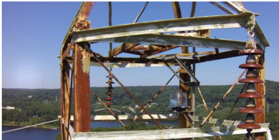
Rusted transmission tower | Eversource Energy
